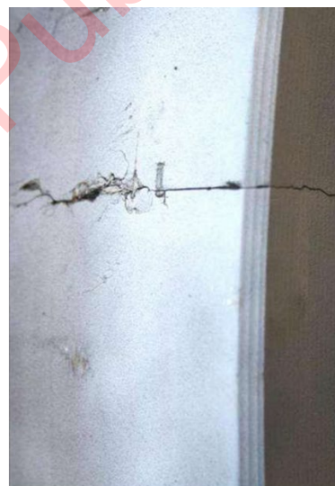
Figure 5:4 – Class 5 Thermal crack
