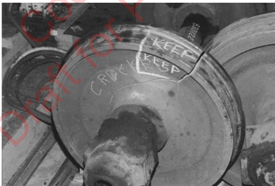
Figure 11:1 – Cracked or broken web
