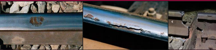
Panoramic data imagery, LiDAR technology, and examples of track defects detected on modern IEVs.
